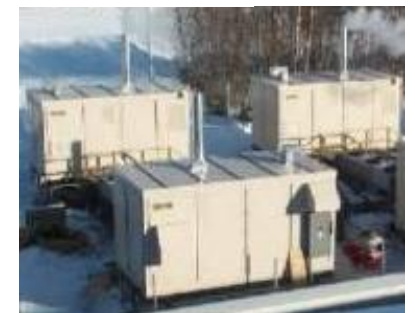
Decentralized & stationary batteries, CH 4 , MeOH, EtOH
